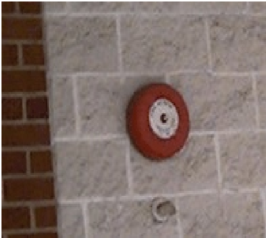
Figure 16 - Sprinkler Alarm Bell
