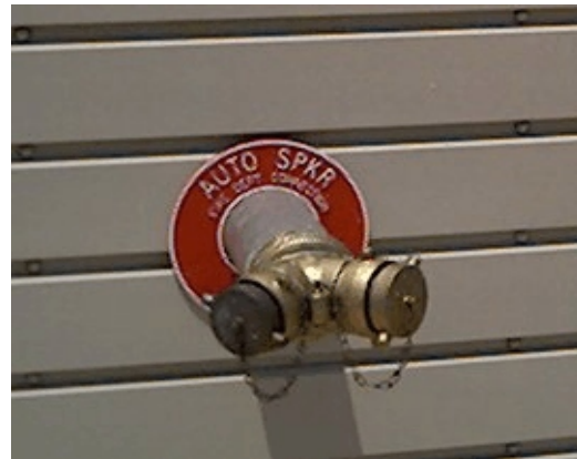
Figure 11 - Fire Department Connection
